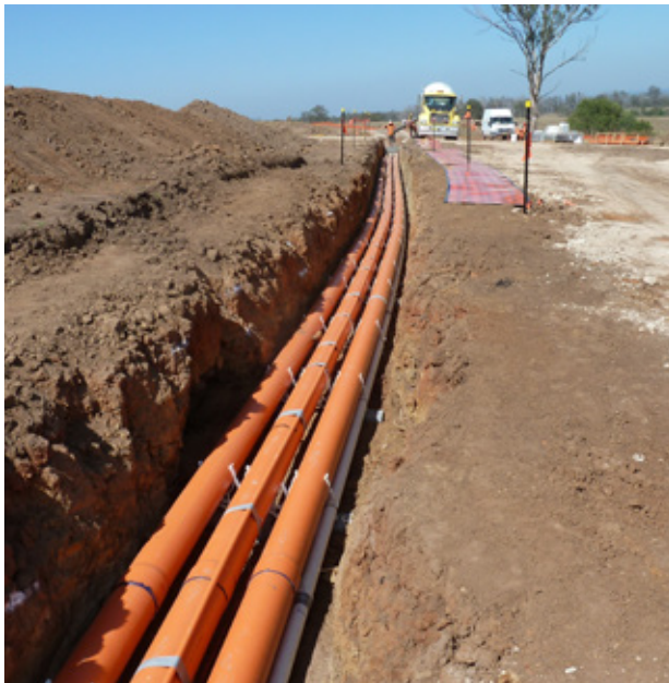
Example cable system installation
