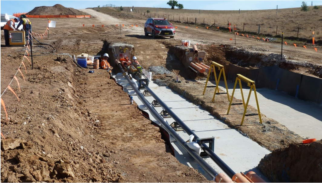
Figure 4-42 Example of a caterpillar pit (Australia)
