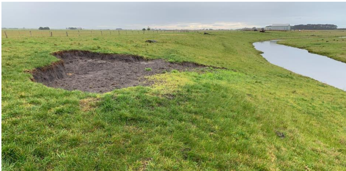
Figure 7-12 Localised erosion on top of the waterway embankment (Photo taken 14/07/2021)
